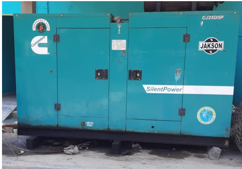
POWER BACKUP SYSTEM
